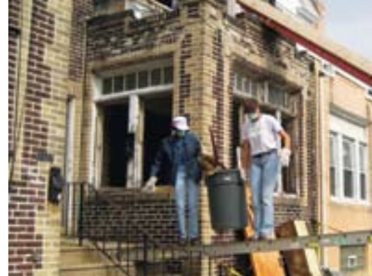
Campbell volunteers help renovate a Camden home for the St. Joseph's Carpenter Society.
