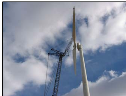
Wray School District Wind Turbine, Wray CO
