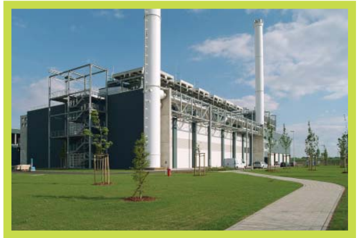
EVC 2 is the specially designed trigeneration facility designed to supply electricity, heating, and cooling to Fab 36 in Dresden, Germany, with a total average efficiency of almost 82 percent. Source: M+W Zander ( www.mw-zander.com ).
