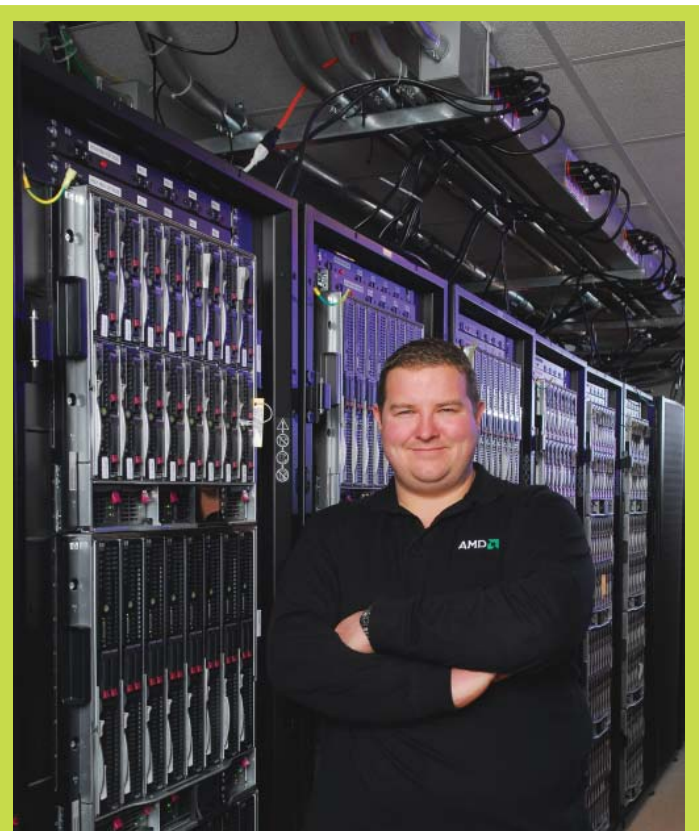
Richard Conohan, Program Manager, AMD Environmental, Health & Safety in a server room at AMD Markham.
