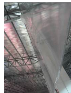
Figure 2. Air curtain installed to increase air flow
