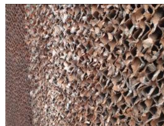
Figure 1. Corroded metal fins of cooling system
